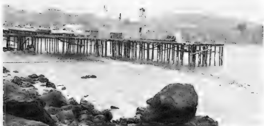
FIG. 3 - END OF DOCK, SHOWING THE DERRICK AND A PILE DRIVER. (THE CABLE IS THE SAME ONE THAT IS SHOWN IN FIG. 1.)
