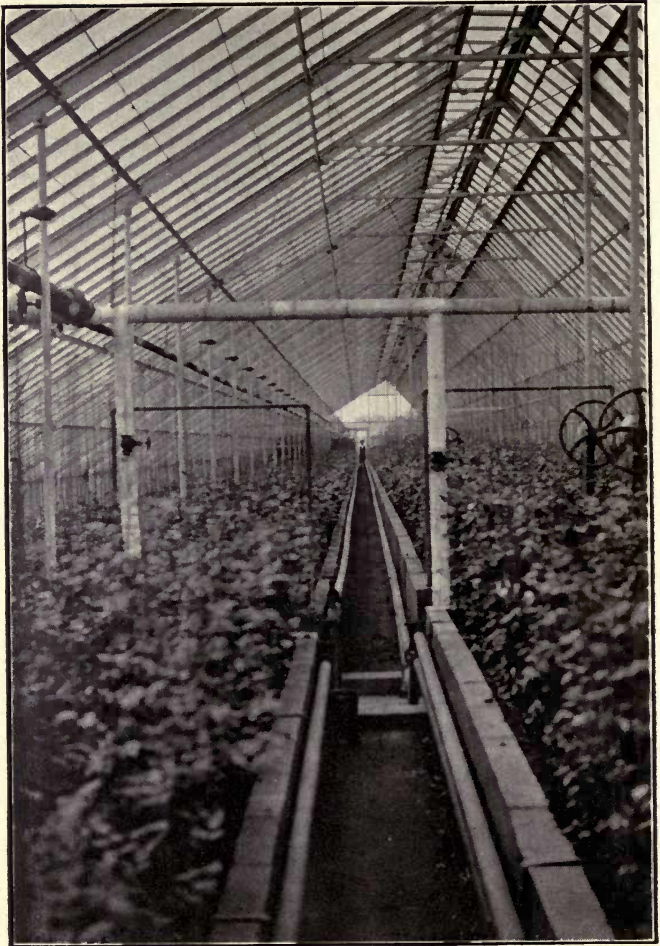
Interior of Rose house showing hot water heating system Courtesy Kroeschell Bros. Co., Chicago, Ill.
