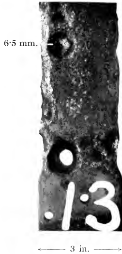
3.75 PER CENT. NICKEL STEEL (K 13) EXPOSED TO HALF-TIDE CONDITIONS AT COLOMBO FOR 5 YEARS, SHOWING HOLE 3 MM. IN DIAMETER NEAR LOWER END, AND VERY DEEP PIT VERTICALLY ABOVE IT.
