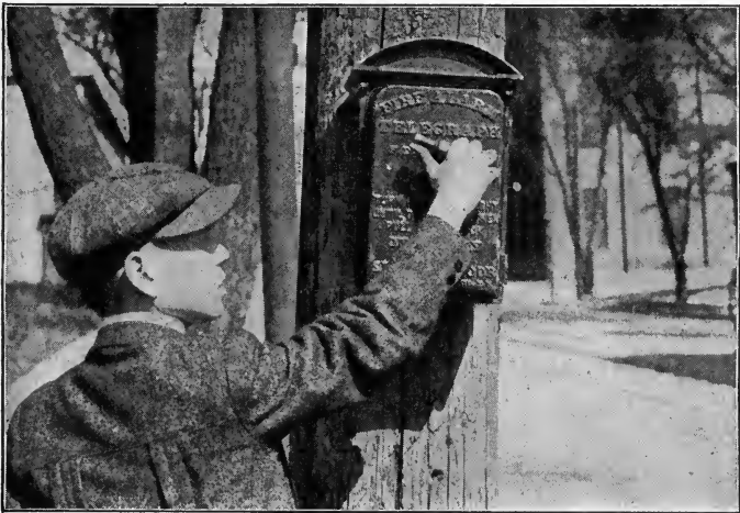
THESE BOXES ARE CONNECTED BY WIRE WITH A CENTRAL EXCHANGE, AND FROM THIS OFFICE THE ALARM IS SENT TO THE COMPANY WHICH IS TO RESPOND
