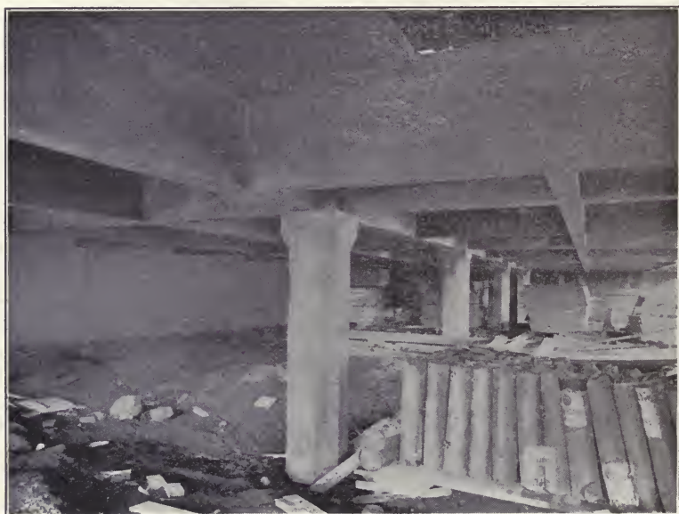
Photo No. 273. DETAILS OF PIERS AND FLOOR BEAMS UNDER HORSE BARN, GEDNEY FARMS, WHITE PLAINS, N. Y.
