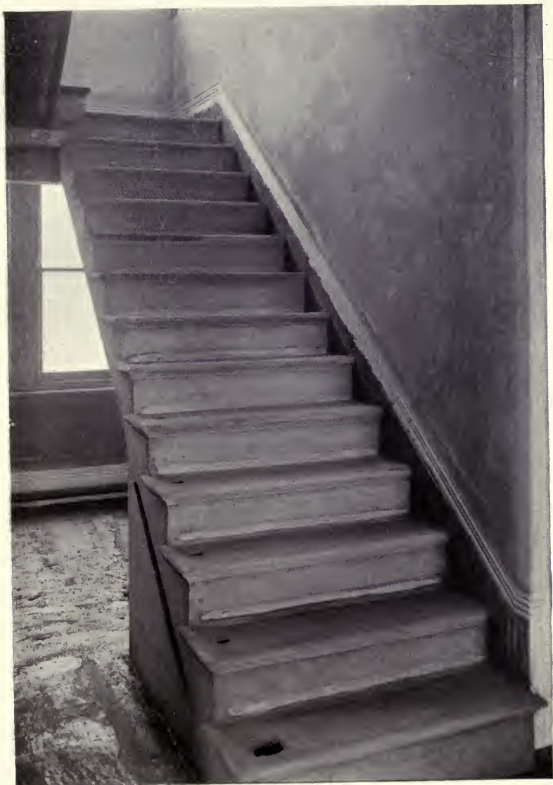
Fig. 17.—Illustration of Stairs, showing holes left for newel and balustrade. The wood insertion for fixing stair-rod eyelets can be seen.
