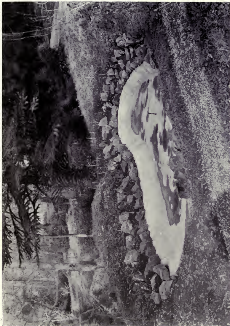
Fig. 14.—A sound 'concrete basin,' bottom and sides reinforced with old iron. (This pond is on a very bad foundation.)
