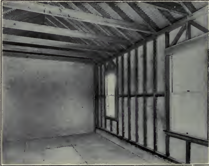
Interior of Garage at Allentown, Showing Wood Frame with Stucco on Both Sides of Metal Lath.
