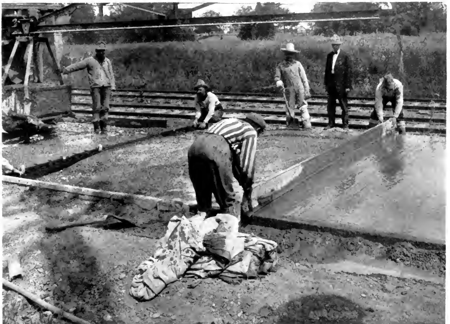
FIG. 47.—USING THE SIDE FORMS AS TRACKS FOR TEMPLLET. Steel Joint Protection Plate Shown at the Left.
