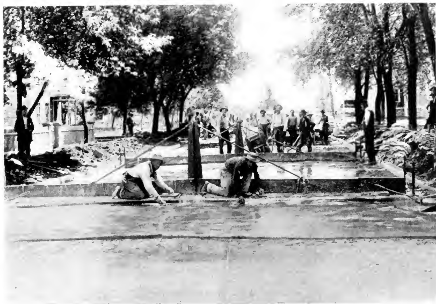
FIG. 37.—DOTY ST., FOND DU LAC, WIS. Finishers working from Roughen's Adjustable Street Gauge
