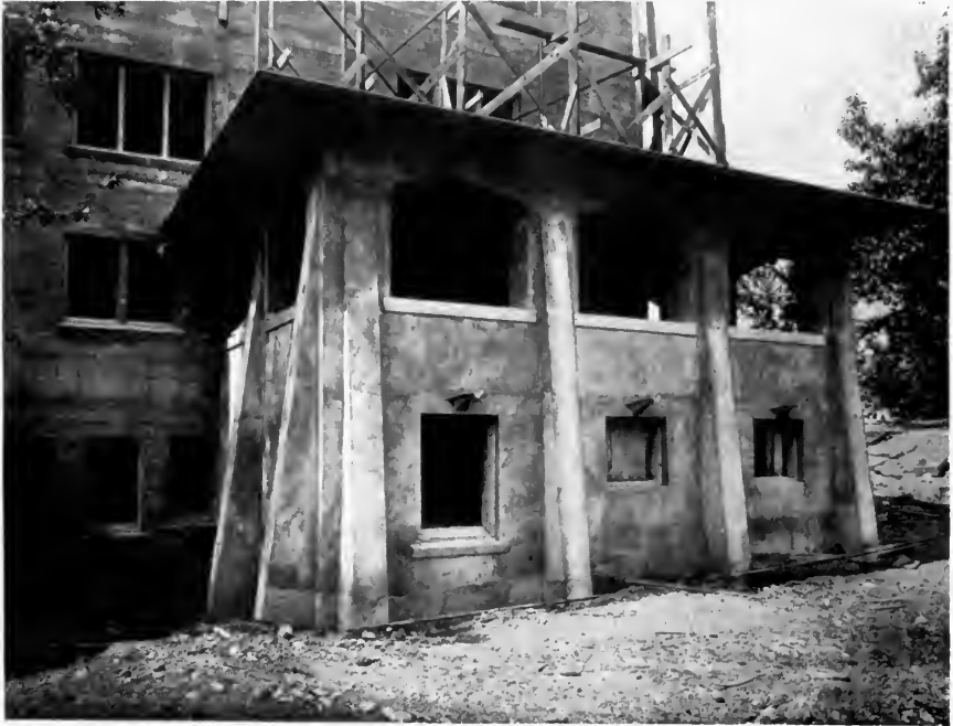
Fig. 4.—Buttressed porch construction in monolithic concrete. Impracticable in other types of masonry.
