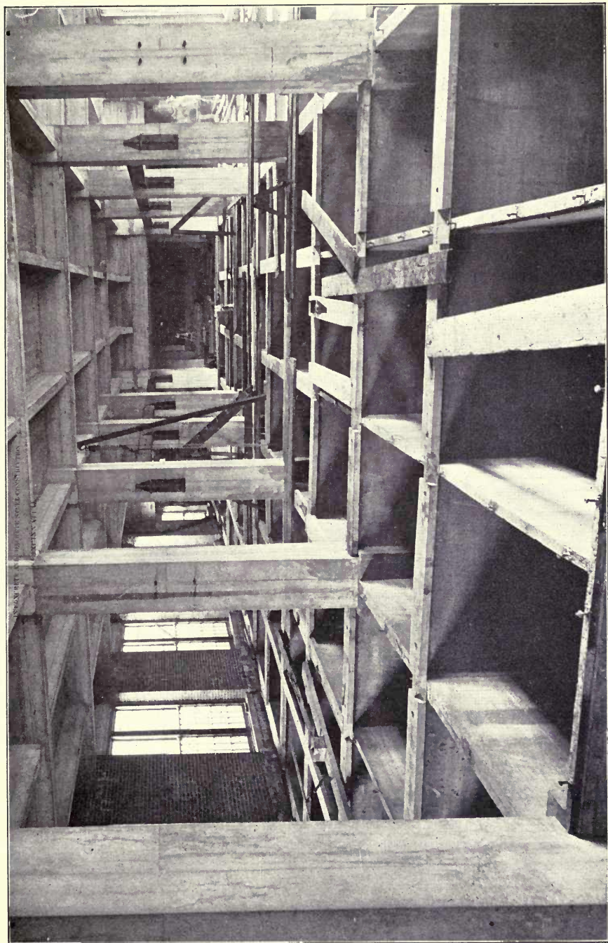
Fig. 134.—Concrete Tanks in American Oak Leather Company Factory. (See p. 202.)
