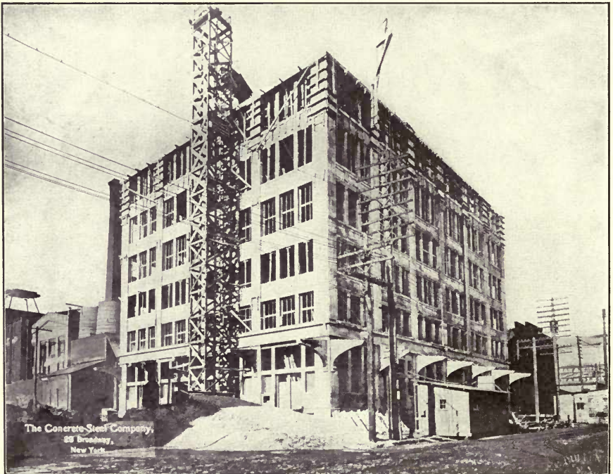
COLGATE SOAP FACTORY, JERSEY CITY, N. J. Dimensions 85 ft. by 104 ft. William P. Field, Chief Engineer; The Concrete-Steel Co., Builders.
