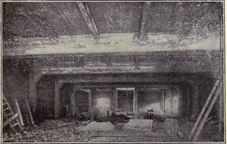
Fig. 329.—Interior View, Robbins Garage, New York City, Showing Floor Girders and Columns.
