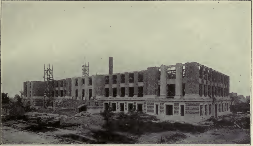
FIG. 8.—NORFOLK HIGH SCHOOL UNDER CONSTRUCTION. REINFORCED CONCRETE SKELETON AND FLOORS WITH BRICK VENEER.
