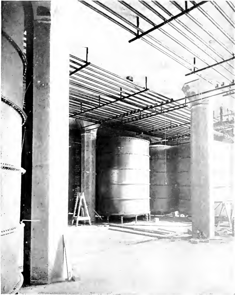
Fig. 17. Interior Stock House Hamm Brewing Company Building, showing 50 ton tanks being placed in position covering full area of floor.
