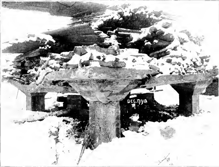
Fig. 71. Failure of Mushroom Slab.
