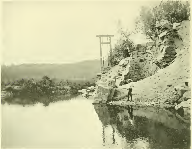
THE BROKEN DAM.
