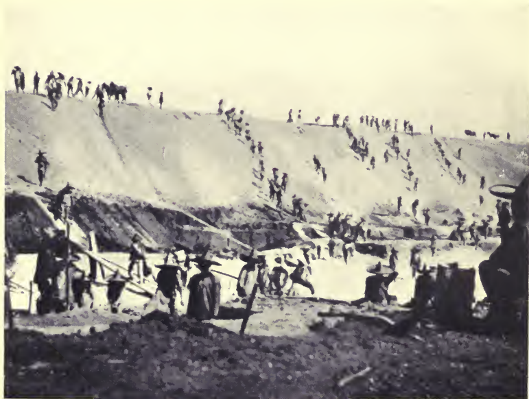
BUILDING THE EARTH RESERVOIR TO RECEIVE THE FLOW FROM POTRERO DE LLANO NO. 4.
