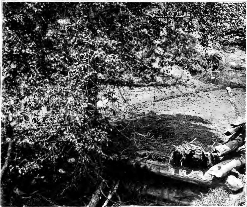
Dam filled with silt, in the Tonto Basin, Arizona—Tonto National Forest will prevent such occurrences in future
