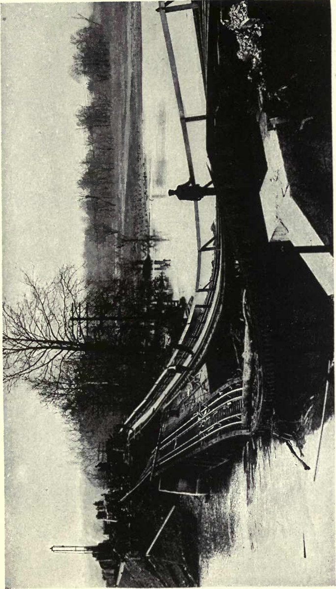
FIG. 84. BRIDGE No. 145, EASTERN DIVISION, OVER BLACK FORK Pier and both embankments badly damaged, 100 feet of embankment washed out
