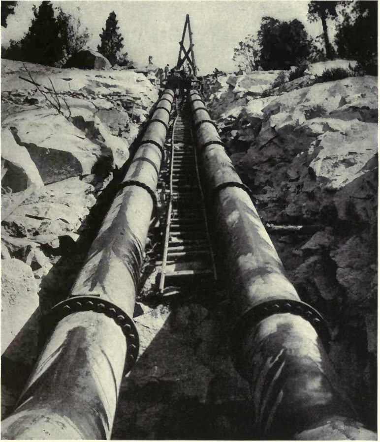
FIG. 55. LAYING PENSTOCK ON 80% GRADE—BIG CREEK DEVELOPMENT PACIFIC LIGHT AND POWER CORP., LOS ANGELES, CAL. (Stone and Webster Eng. Corp.)
