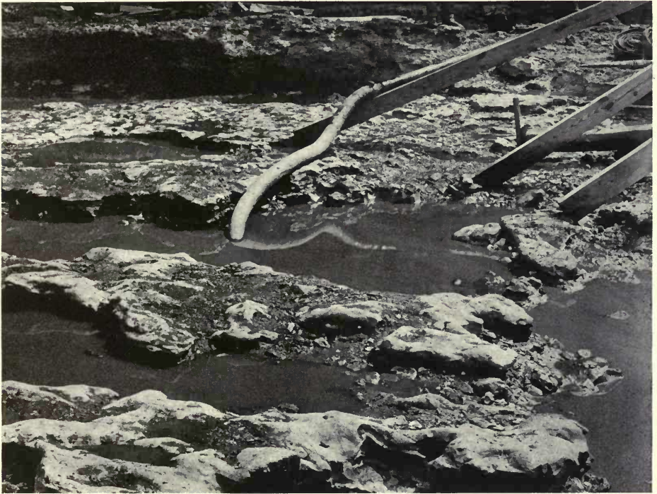
FIG. 22. MISSISSIPPI RIVER POWER CO. RIVER BED EXPOSED IN CONSTRUCTING DAM AT KEOKUK (Stone and Webster Eng. Corp.)
