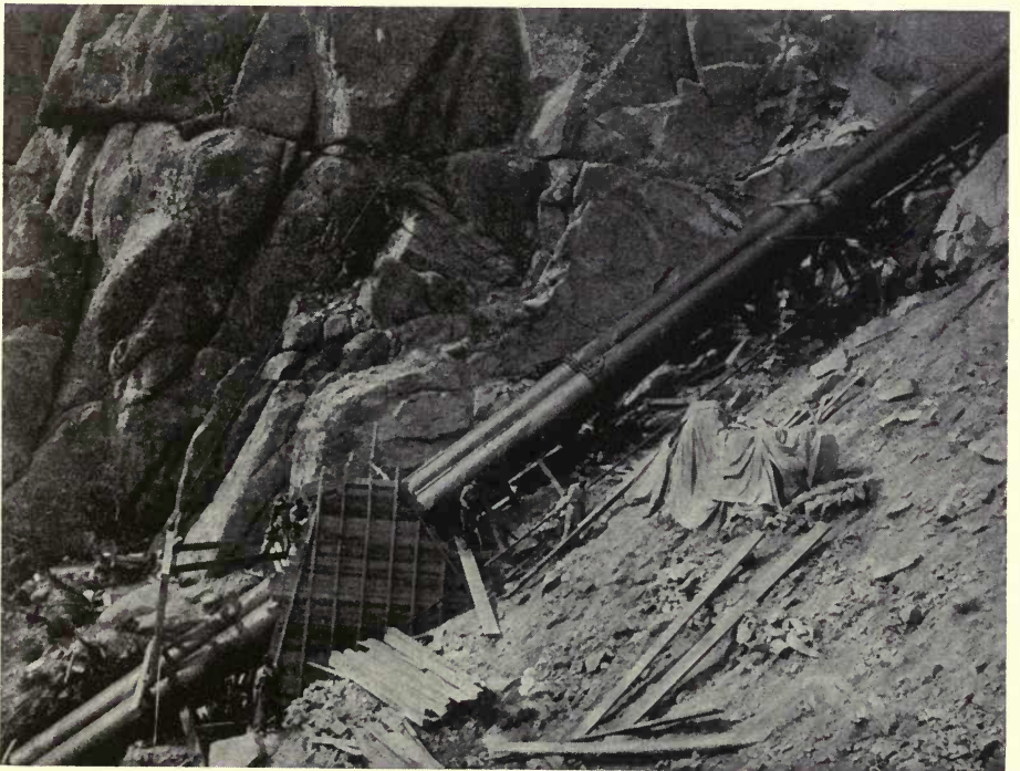
FIG. 54. PLACING FORMS FOR ANCHORS TO PENSTOCK—BIG CREEK DEVELOPMENT PACIFIC LIGHT AND POWER CORP., LOS ANGELES, CAL. (Stone and Webster Eng. Corp.)
