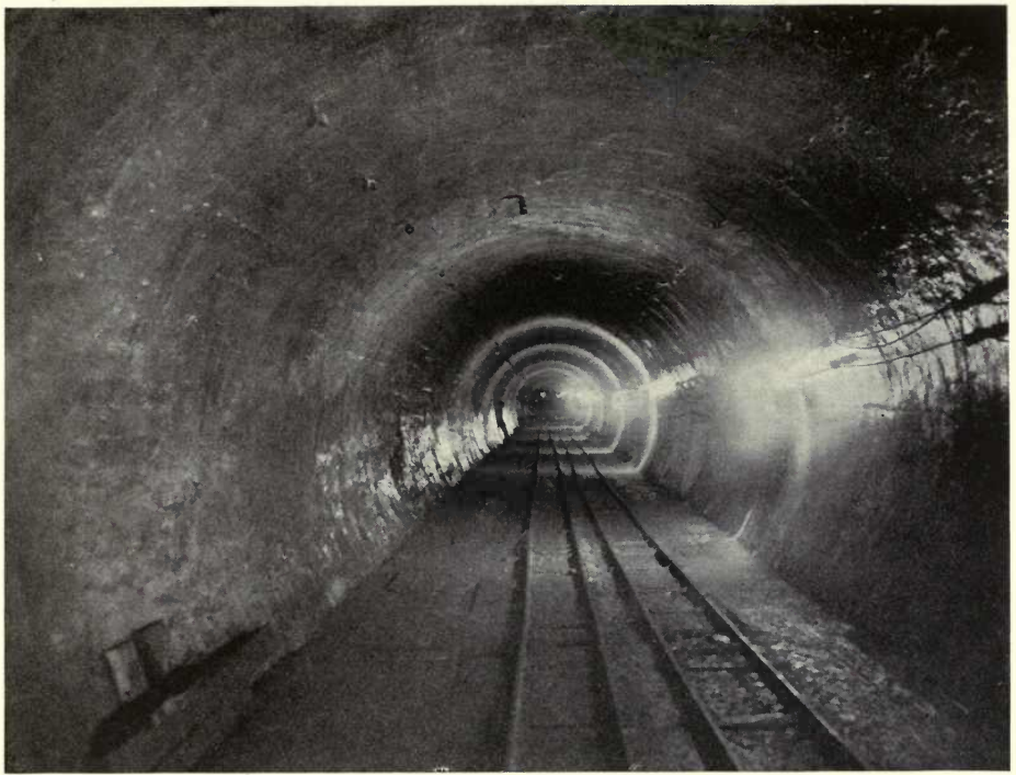
FIG. 51. YUMA PROJECT, ARIZONA-CALIFORNIA SIPHON UNDER COLORADO RIVER—1000 feet long, 14 feet diameter (U. S. Reclamation Service)
