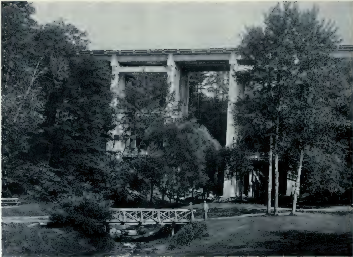
BRIDGE NO. 0.9, ONE OF TWO NEW VIADUCTS BUILT BY THE C.P.R. ON THE NEW SUBDIVISION BETWEEN LEASIDE AND TORONTO.
