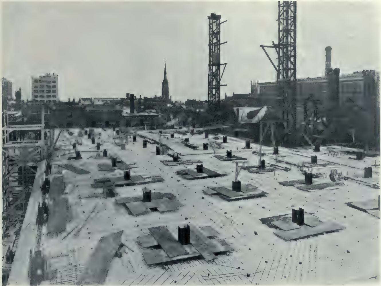
VIEW SHOWING SLAB REINFORCEMENT AND STEEL CORES OF COLUMNS, THE T. EATON COMPANY'S NEW FACTORY, TORONTO.
