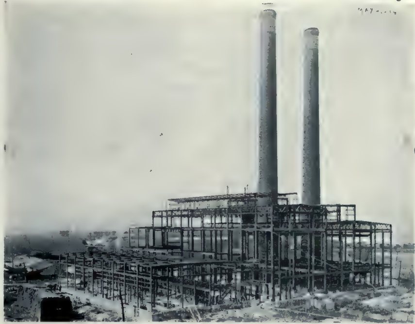
DOMINION POWER AND TRANSMISSION COMPANY PLANT, SHOWING STEEL FRAME AT TIME OF ERECTION.
