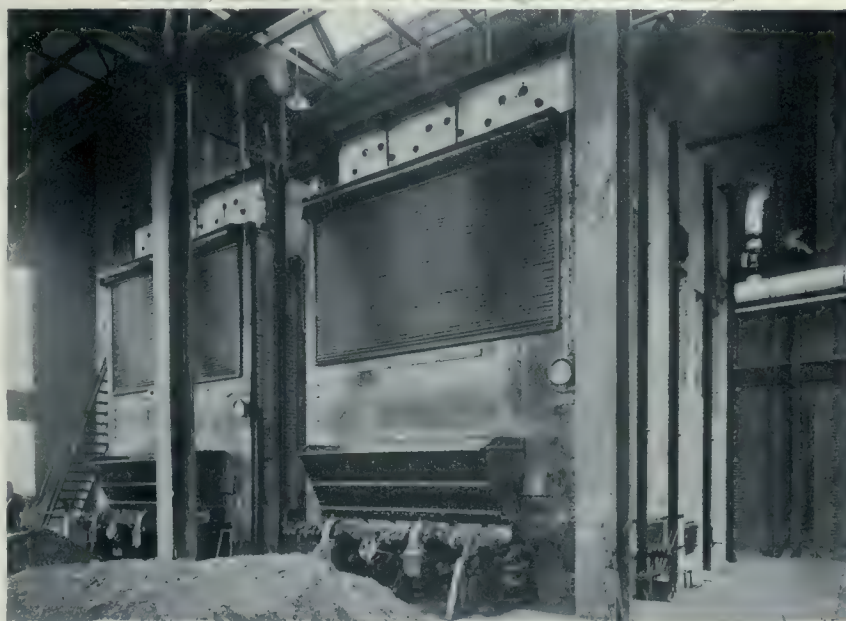
BOILER ROOM, GOODYEAR TIRE AND RUBBER COMPANY'S NEW FACTORY.
