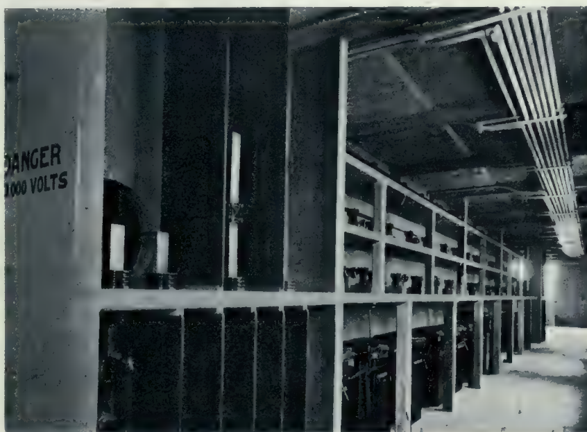
PARTIAL VIEW OF 6,600 VOLT BUS STRUCTURE.
