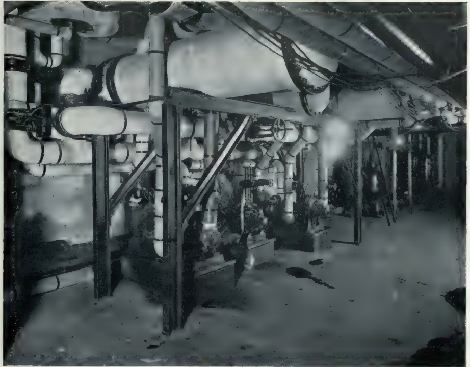
HEATING APPARATUS AND CIRCULATING PUMPS.
