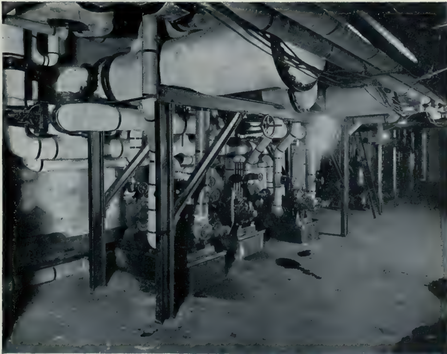
PUMP AND HEATER ROOM, SUN LIFE BUILDING, MONTREAL, QUE.
