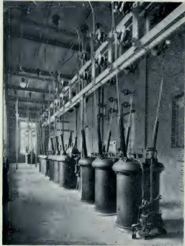
OIL SWITCHES AND BUSES FOR 42,000 VOLT CURRENT.
