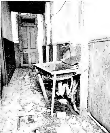
FIG. 100.—A hall and sink as the Department found them.
