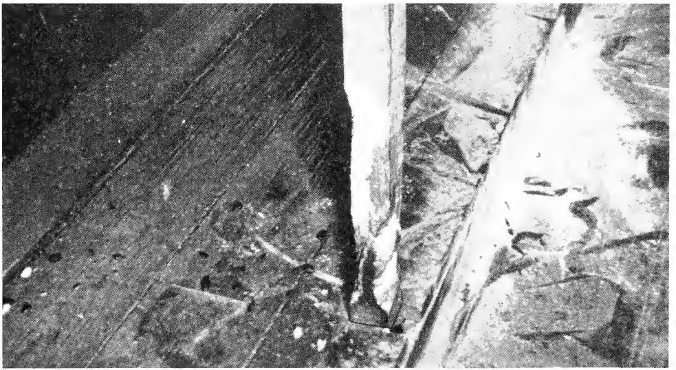
Fig. 4.—Evidences of rats: Droppings and damage to grain sacks; tracks in dust; a freshly gnawed post, and footprints and tail marks in flour. Courtesy of U. S. Public Health Service.
