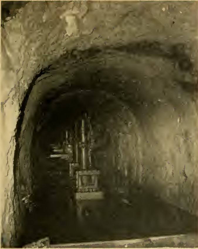
Photo No. 34. Machine tools standing in water. Landslide had formed a dam near entrance.
