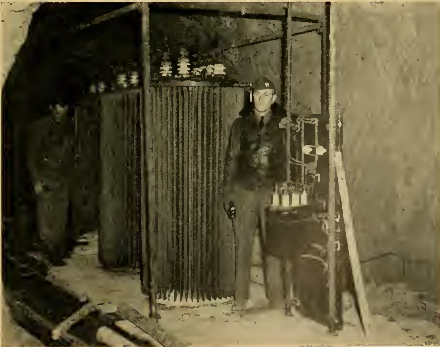
Photo No. 35. Three 250-kv.-a. transformers, Yoshimatsu.
