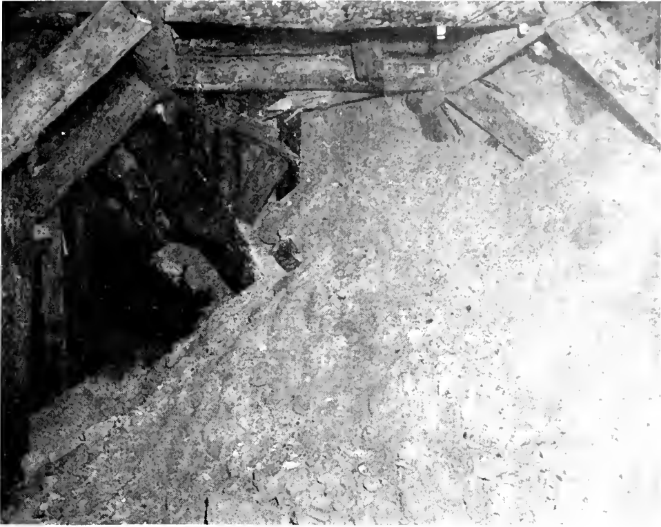
Photo No. 52. Cave-in of machine shop at Seto.
