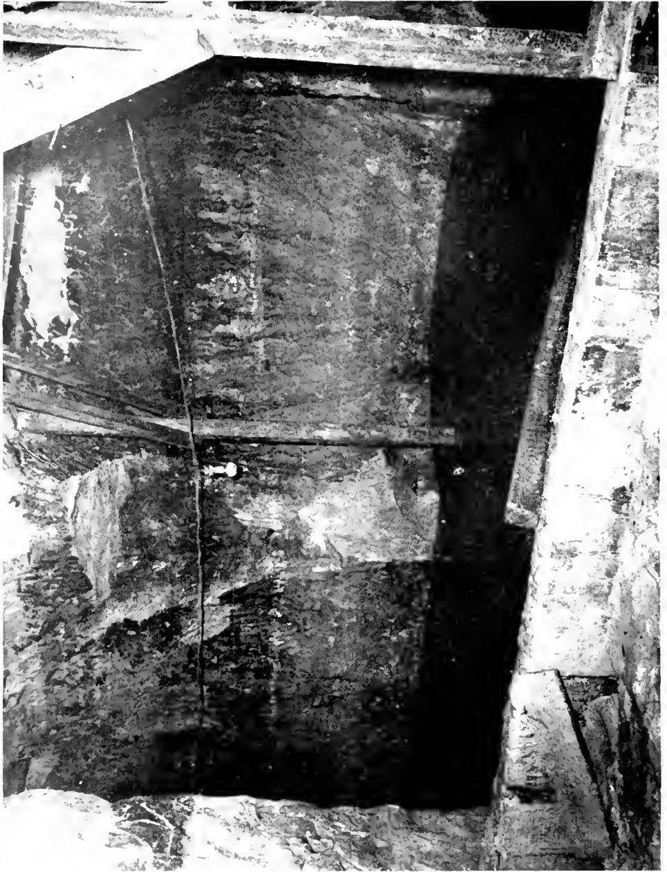
Photo No. 44. Flooded tunnel at Hisai.
