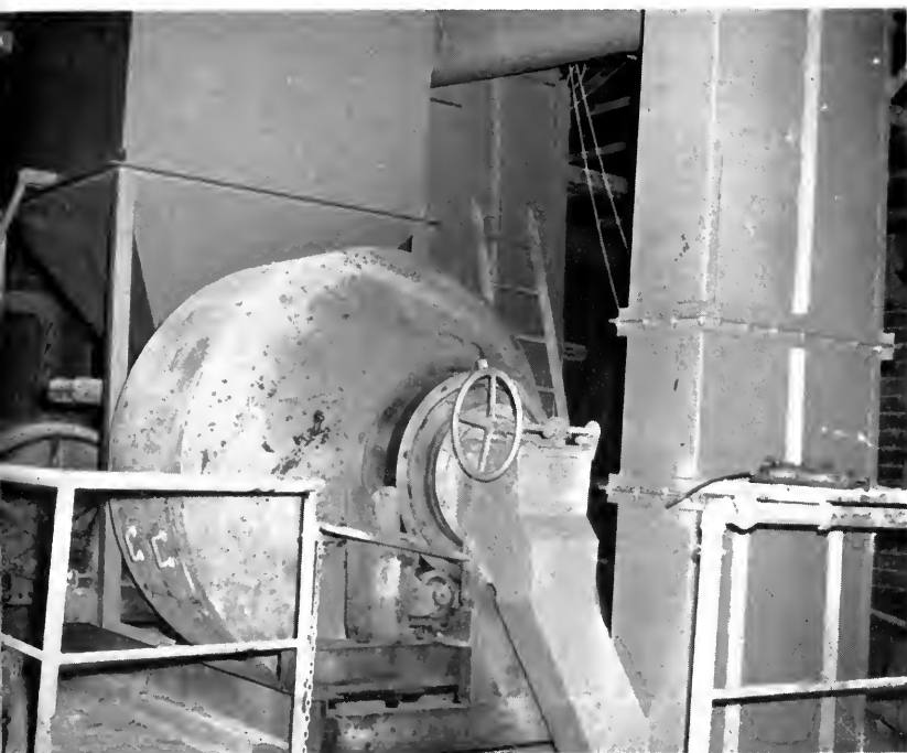
In most combination horizontal-vertical plants, materials flow from the holding bin into the mixer. After mixing, the materials are discharged into an elevator. (Fig. 13)
