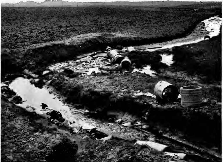
A washed out tile line makes greater inroads each year into farm income. Crops and cropland are lost, and repair becomes more costly. A grass waterway in this natural drainageway would have prevented this gully. Tile seldom work in these slowly permeable soils. (Fig. 17)
