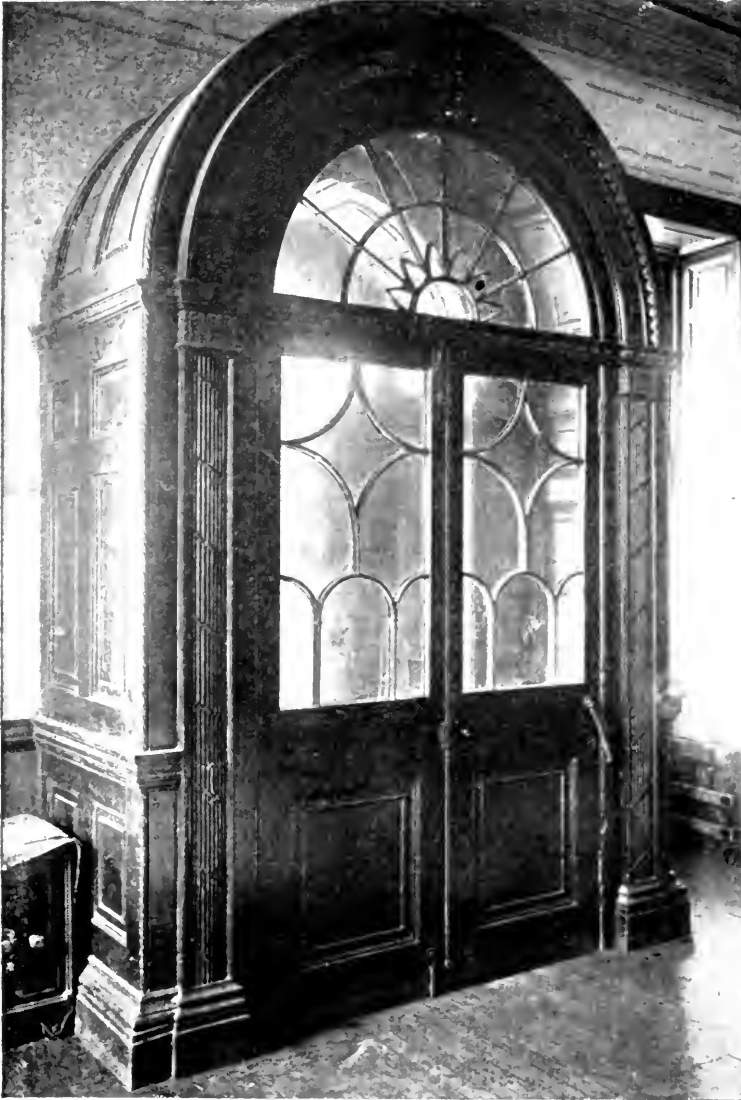
Vestibule door at Alexandria, Va. An interesting treatment, but somewhat difficult to keep clean on top
