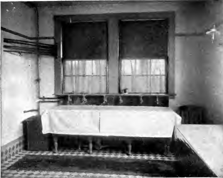
End of a first-story laundry showing the relative position of the soapstone tubs to the light
