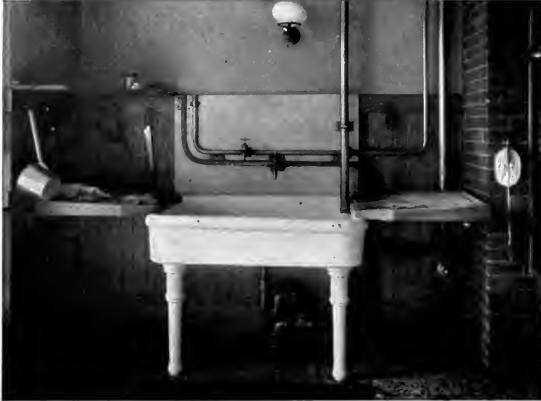
An enamelled kitchen sink with hot and cold water and trapped waste. The overflow or waste which empties into it is after the manner of the ice-chest waste
