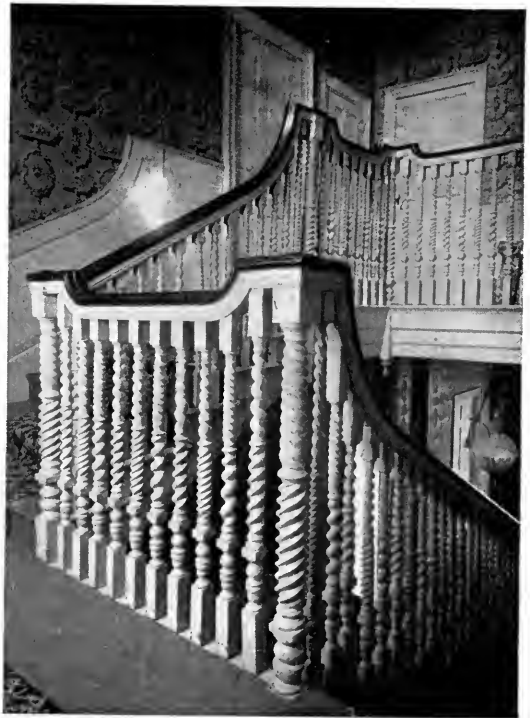
Landing of Jamaica Plain stairs, showing details of post, balusters and rail
