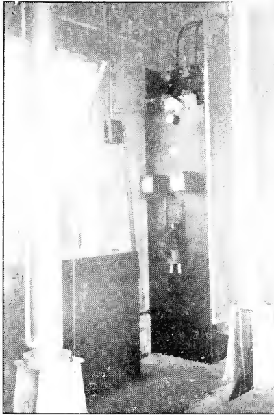
View of Switchboard and Valve Control Desk
