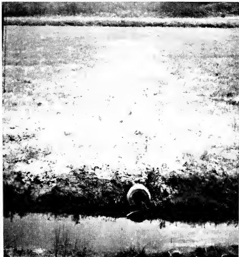
Figure 3. Improving poor drainage with a rock drain (tile only on the ditch end).
