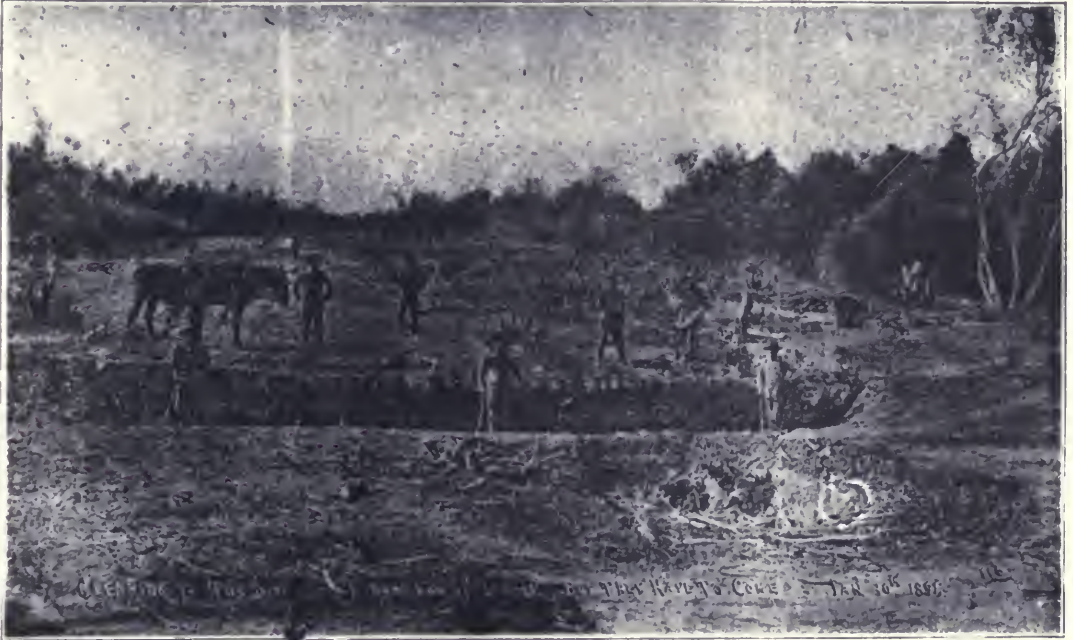
13—The character of the wilderness the crew had to clear one hundred feet wide for seven miles. The stumps had to be cut out for about one-half that width. The chaparral is mostly acacia, which is a hard and close grained wood, and has many long roots. The tree and roots are excellent for charcoal and 'o fuel—equal, probably, to hickory. This Ditchway has been cleared 100 feet wide from the tail gate, fourteen miles, to Pacific City site.
