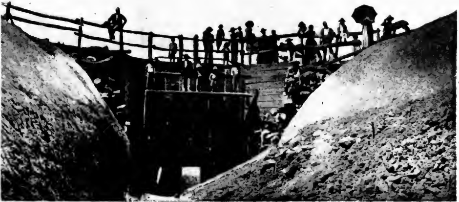
The temporary head gate and bridge at a quarter of a mile below the point where the permanent head gate will be. The ditch is about twenty feet deep at this point but when this photograph was taken, May, 1892, the scrapings from the sides were still at the bottom. Friend Victor C. Mikes stands at the gate opening on the loose earth. The river rises about fifteen feet during floods and this gate is to control it from smothering out our own farms by w
