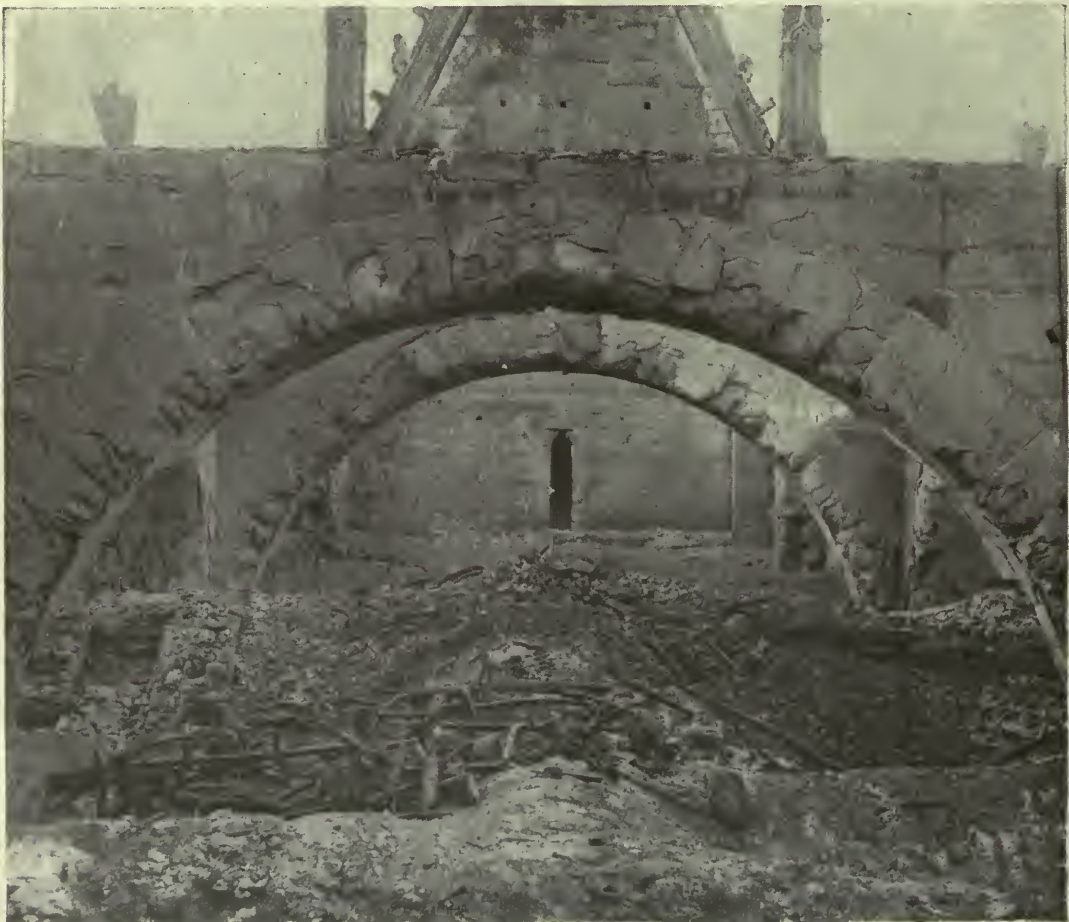
WRECKAGE OF THE ROOF.
