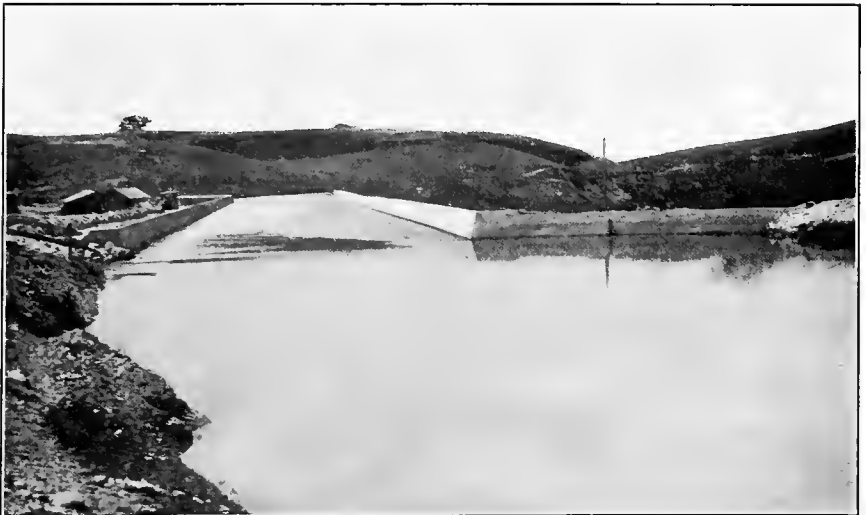
FIG. B.—Lined canal on hydraulic fill used to replace wood flume, Turlock Irrigation District.
