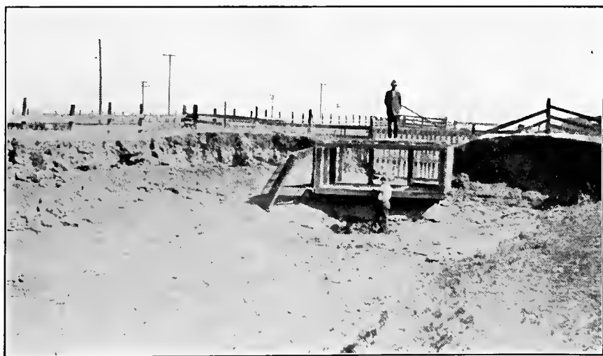
FIG. B.—Erosion below structure.
