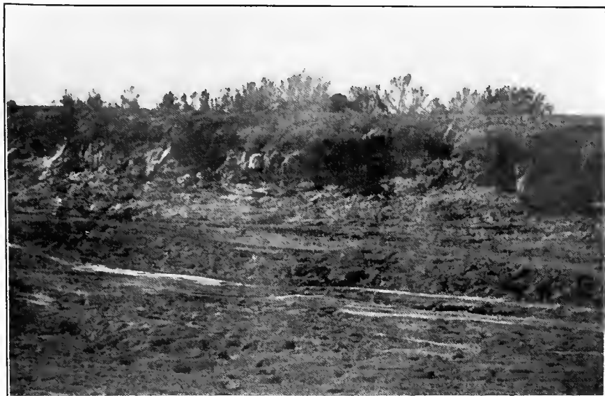
FIG. A.—Eroded bank in sandy soil before lining, Main canal, Minidoka project.
