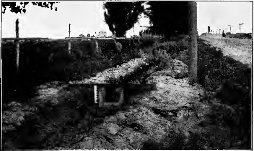
FIG. B.—Weir with gage graduated to read discharge directly, Twin Falls Salmon River System.
