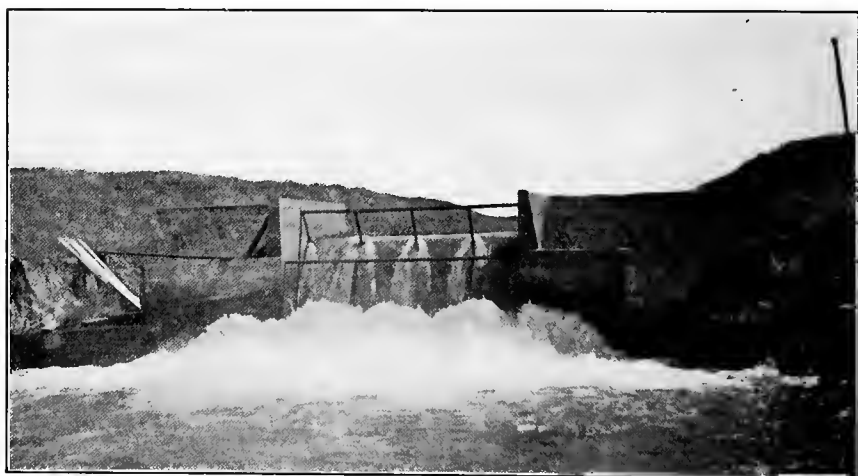
FIG. D.—Erosion below drop, Modesto irrigation district.
