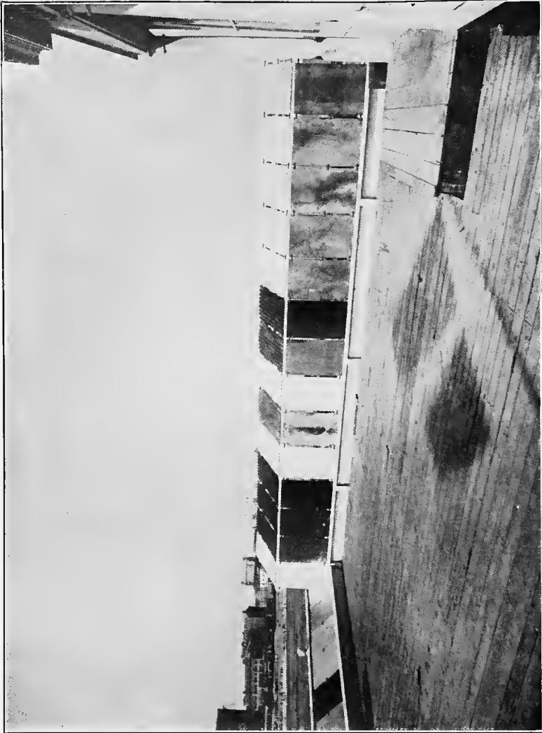
FIG. 64. — Test of galvanized and black iron roofing and sheathing, U. S. Geological Survey, Young's Old Pier, Atlantic City, N. J.
