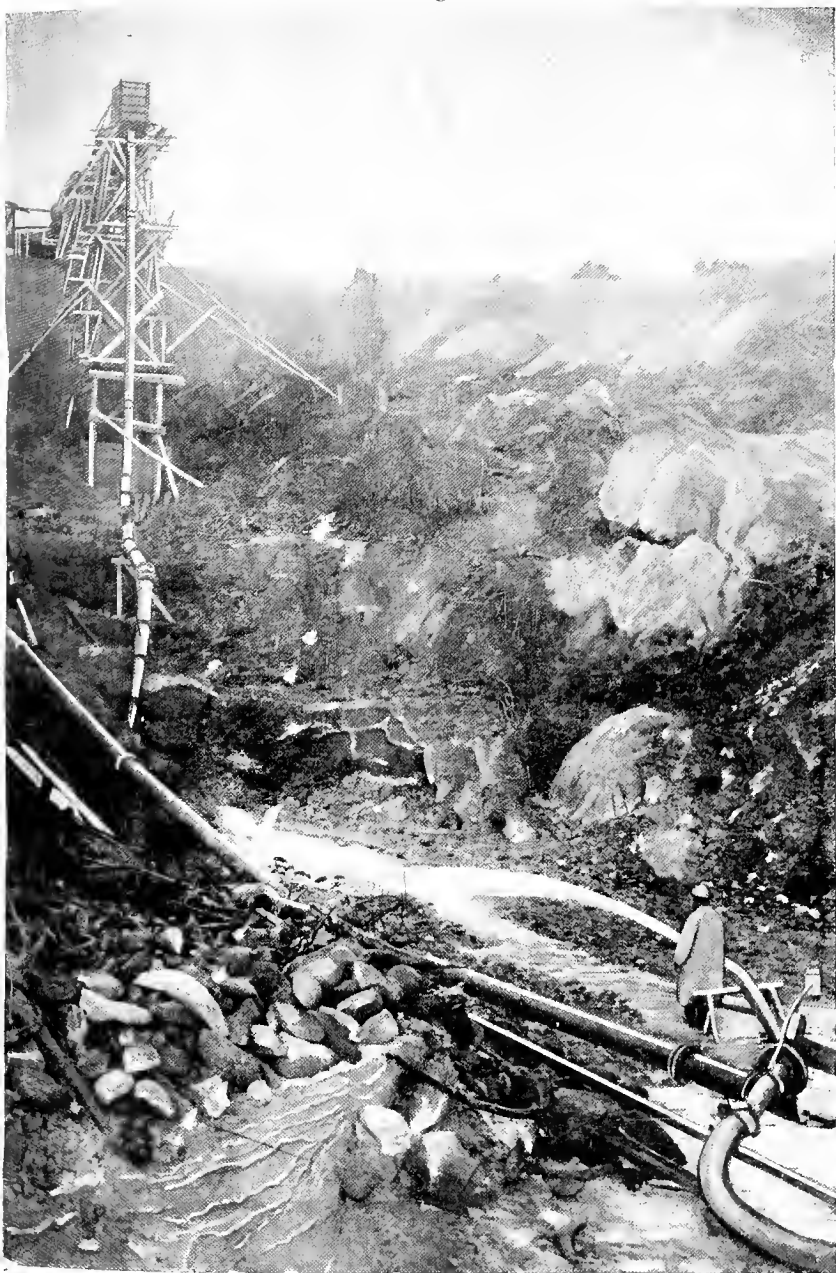
ROUND HILL GOLD-MINING COMPANY: NOZZLES AND HYDRAULIC ELEVATOR. Mining Handbook.
