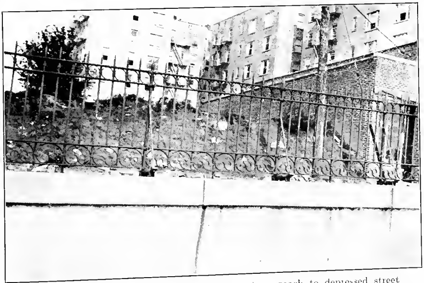
FIG. B.—Picket fence. Wall lining open cut approach to depressed street crossing.
