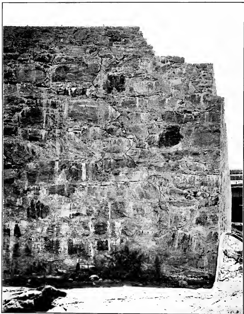
FIG. C.—Crack at sharp corner of wall due to tension component of thrust.
