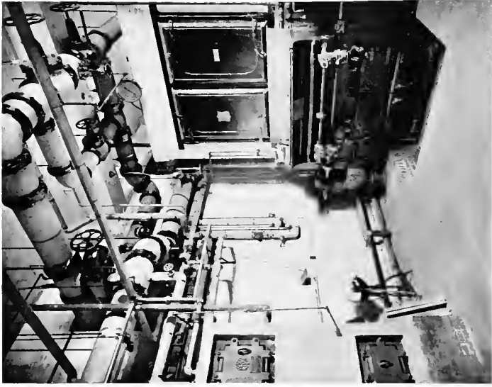
One of the Boilers in the Well-Equipped Engine Room
