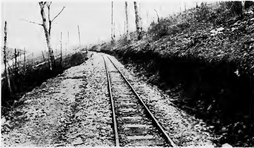
RECONSTRUCTED GERMAN LINE. TRACK CONSTRUCTED BY FIRST BATTALION DURING ST. MIHIEL DRIVE
