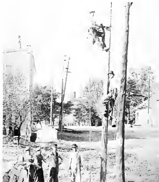
Lights came to Greenup in the summer of 1899. Village employees set poles and strung wire. Note the wooden water tower.
