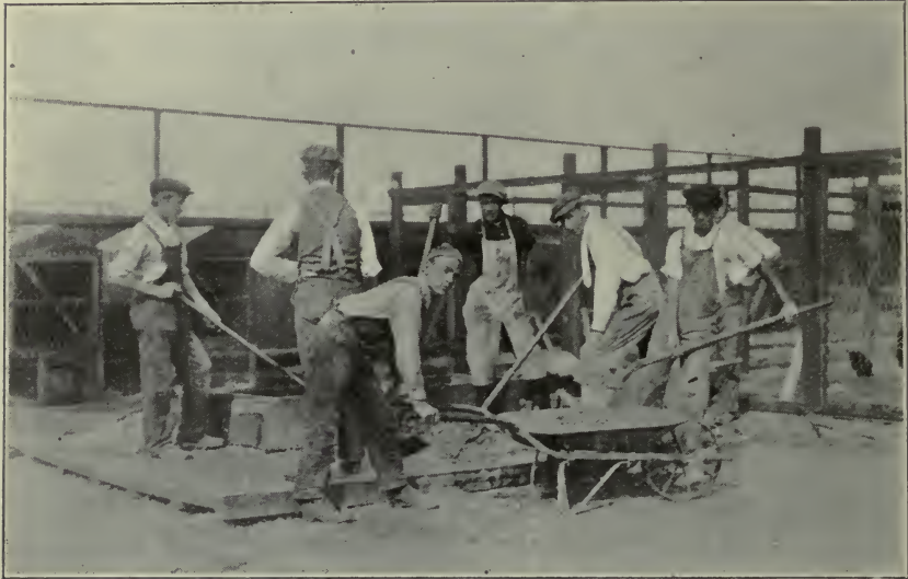
Manual Training and Agriculture: Cementing poultry house floor. Seventh and eighth grade boys.
