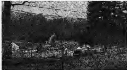
A new residence hall is being constructed on the South Side of campus.
