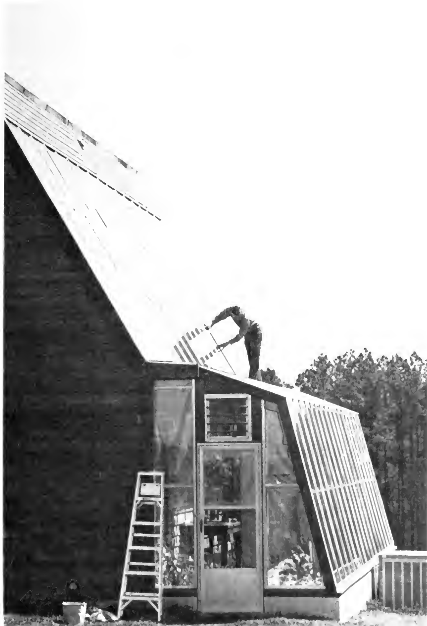
A solar greenhouse and residence.
