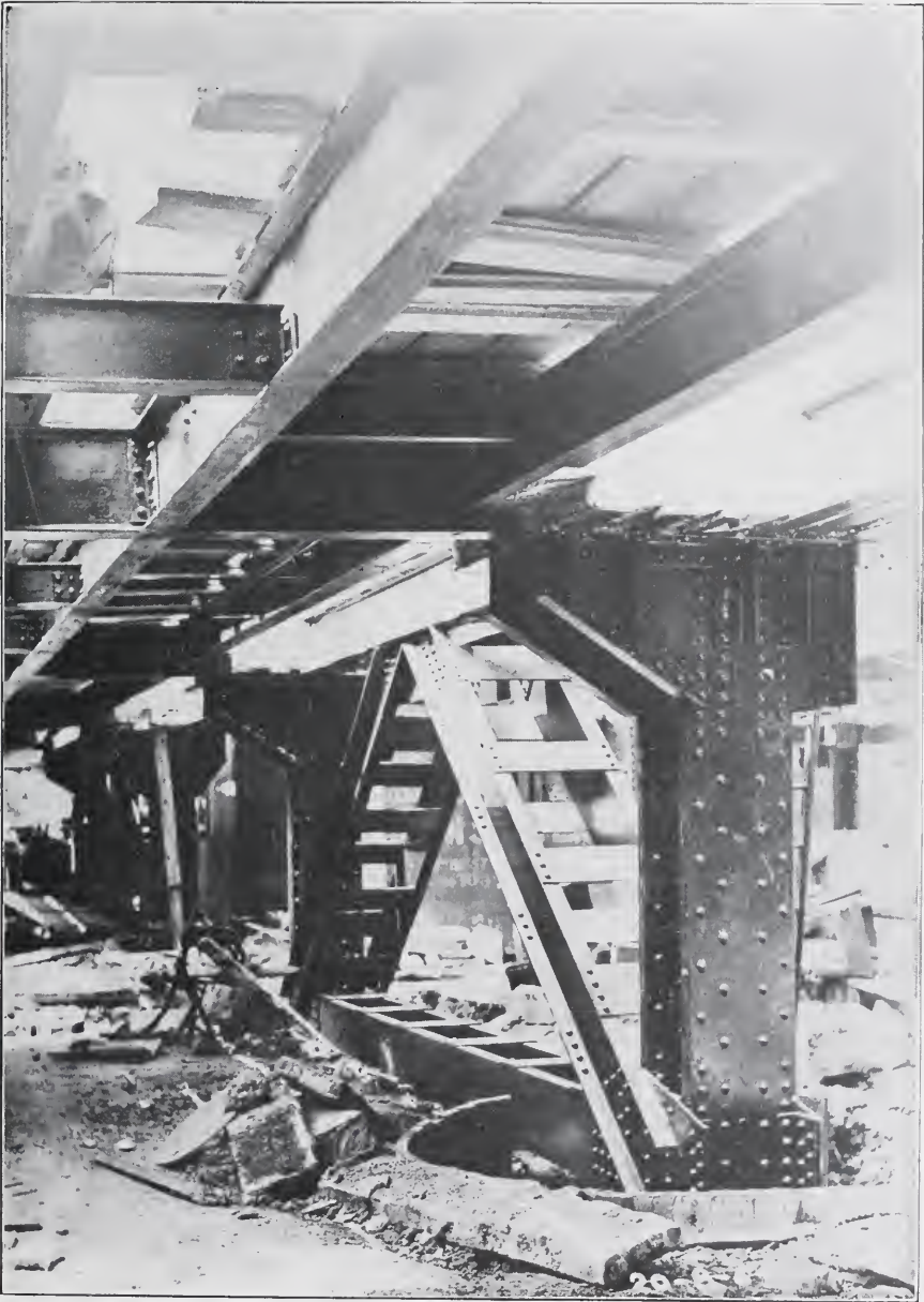
OFFICE BUILDING FOR CHICAGO & NORTHWESTERN RAILWAY COMPANY, CHICAGO Details of wind-bracing construction in basement. Note connection of beams to girders, also girder connection to column. Note that all connections are riveted.
