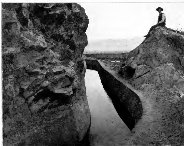
Fig. 5. Completed Portion of Upper Main Canal at Pogue Flats, Okanogan Project, Washington.
