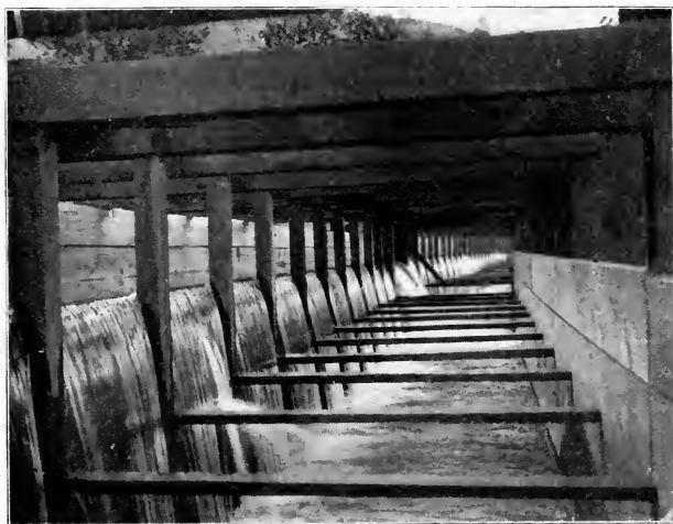
Fig. 12. Interior of Automatic Spillway for Control of Water Supply in Canal on Yakima Project, Washington.
