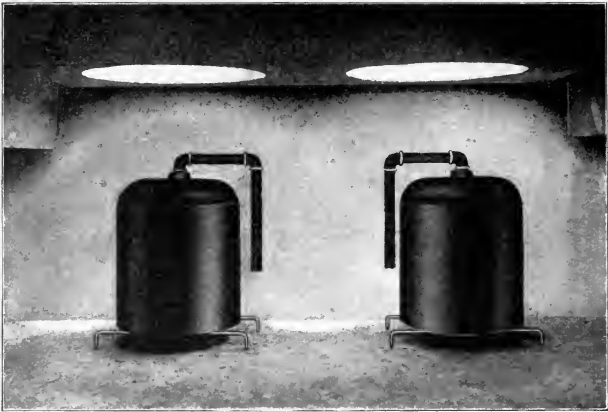
Fig. 46. Interior of "Dosing Chamber" of Septic Tank at Ames, Iowa, Showing "Alternating" Siphons.
