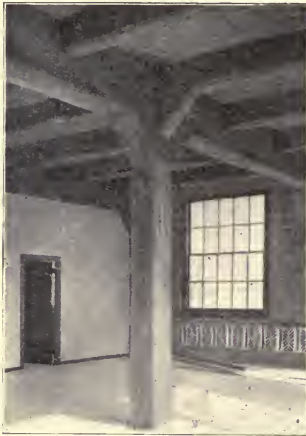
Fig. 203. Floor Construction in Shop Building of Swarthmore (Pa.) College, Showing Connection of Girder Beams with Column.
