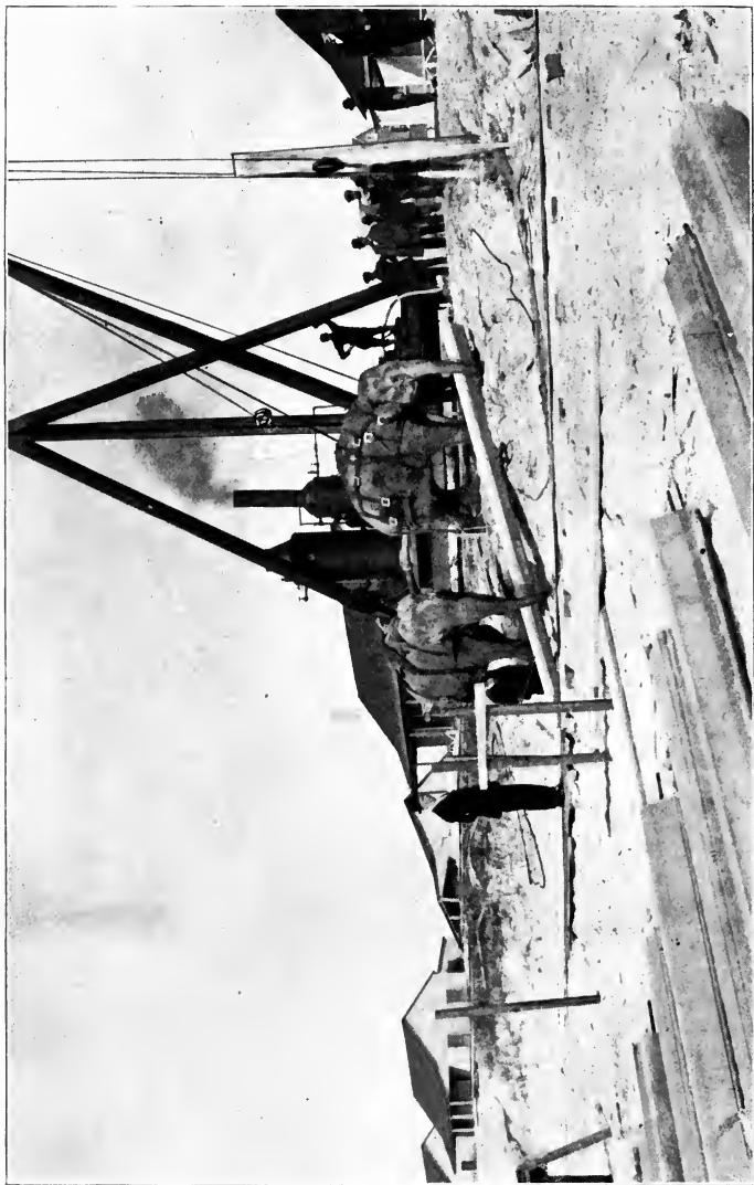
ELEPHANTS CARRYING CONCRETE PILES FOR CONSTRUCTION OF BOARD-WALK AT LONG BEACH, LONG ISLAND, N. Y.
