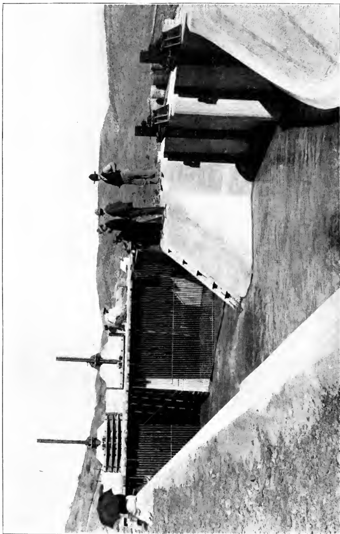
SLUDGE GATES AND ENTRANCE END OF COTTONWOOD PRESSURE PIPE Salt River Project, Arizona.
