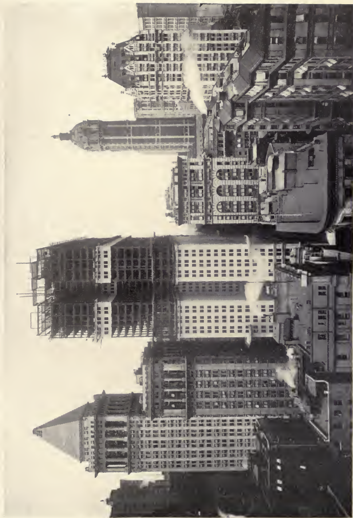
EQUITABLE BUILDING, NEW YORK CITY, IN PROCESS OF CONSTRUCTION Photo by Brown Brothers, New York City
