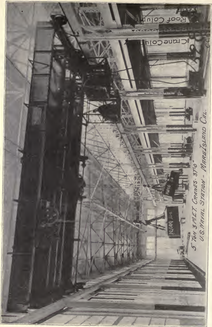
Fig. 117. Five-Ton Electric Traveling Cranes Installed at U. S. Naval Station, Mare Island, California. Courtesy of Cleveland Crane & Car Company, Cleveland, Ohio.
