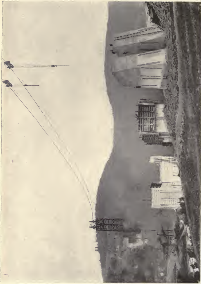
CONSTRUCTING REINFORCED CONCRETE PIERS FOR THE TUNKHANNOCK CREEK VIADUCT ON THE DELAWARE, LACKAWANNA, AND WESTERN RAILROAD
