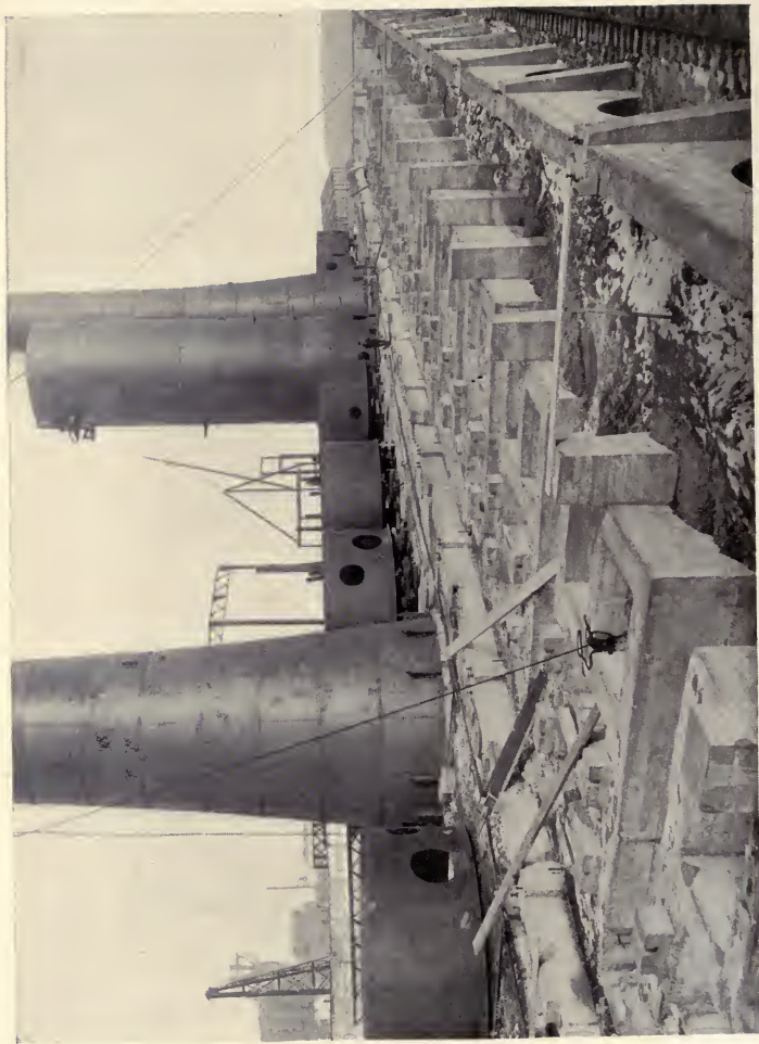
FOUNDATION WORK OF BLAST FURNACES FOR THE IROQUOIS IRON COMPANY 18,000 concrete piles are driven and 35,000 cubic yards of concrete are placed in ten months. Courtesy of Great Lakes Dredge and Dock Company, Chicago
