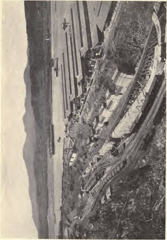
GENERAL VIEW OF DRY DOCK No. 1 IN PROCESS OF CONSTRUCTION AT BALBOA TERMINALS
