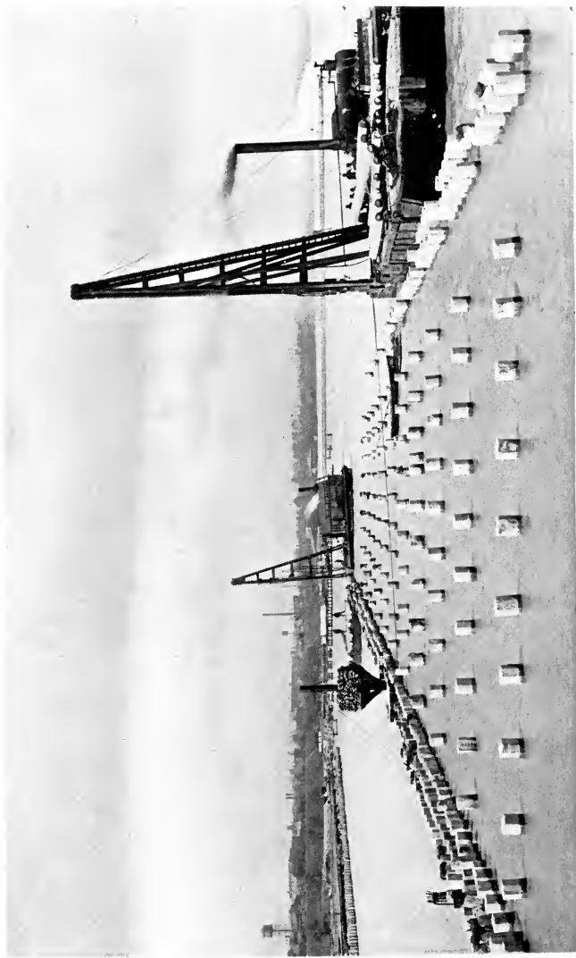
REINFORCED CONCRETE PILES IN PLACE AS SUB-STRUCTURE FOR ORE DOCK A 50-ton test load of pig iron has been mounted on one pile to show whether any appreciable settling resulted. Courtesy of Great Lakes Dredge and Dock Company, Chicago
