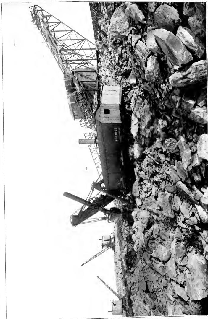
HANDLING ROCK ON THE NEW YORK STATE BARGE CANAL A Bueyrus 70-ton shovel on rock excavator on the line of the canal.
