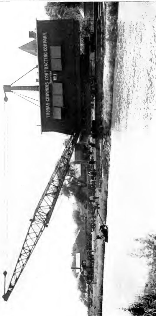
LIDGERWOOD-CRAWFORD SCRAPER BUCKET EXCAVATOR Courtesy of Lidgerwood Manufacturing Company, New York City
