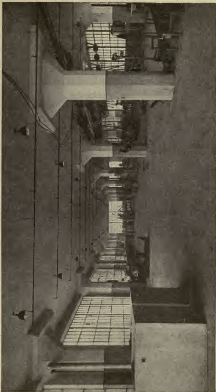
Fig. 214. Interior of H. T. Heinz Company Warehouse, Showing Example of Flat-Slab Ceiling Construction Courtesy of The Condron Company, Chicago
