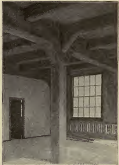
Fig. 212. Floor Construction in Shop Building of Swarthmore (Pa.) College Showing Connection of Girder Beams with Column
