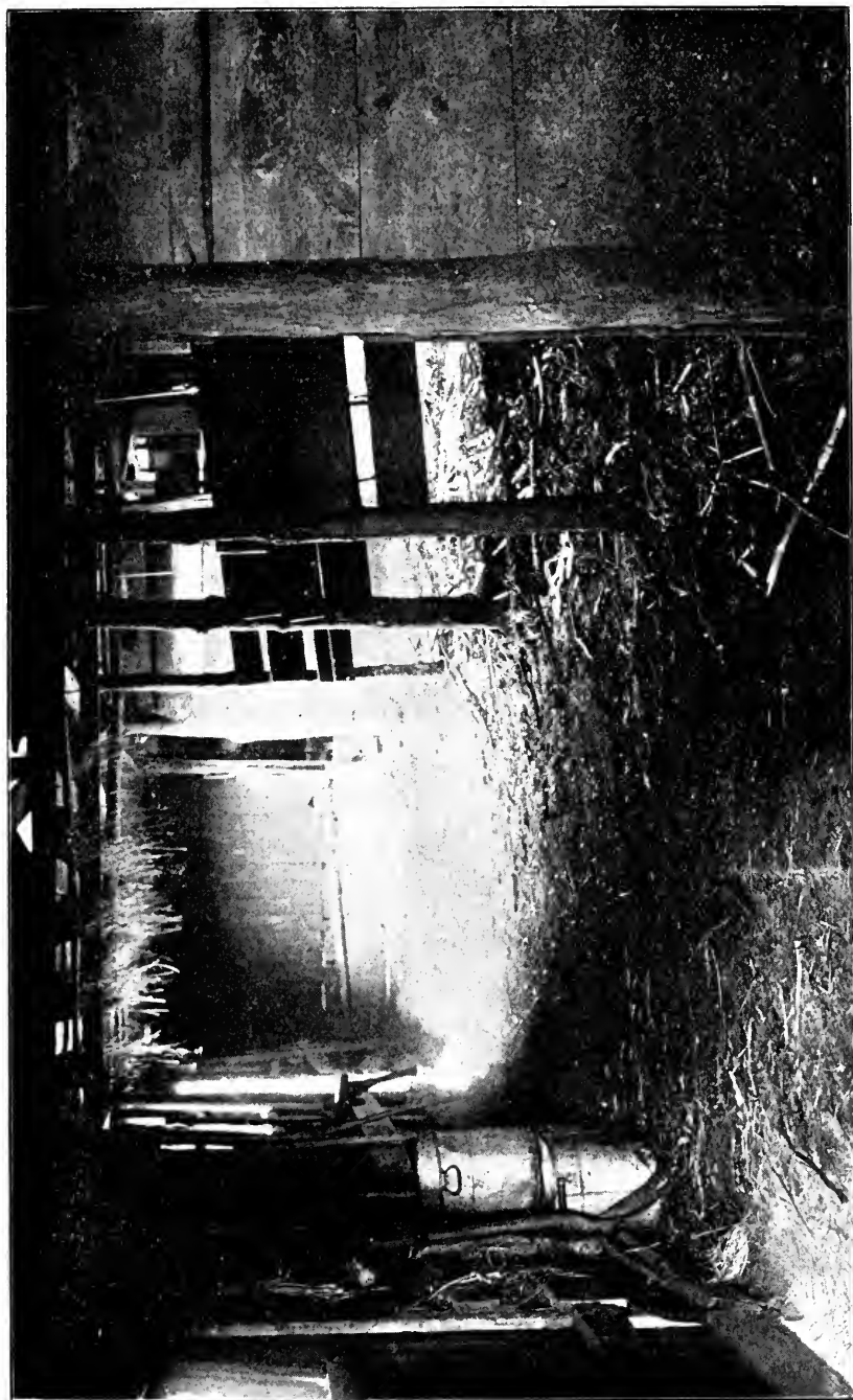
CUT 23. WHILE THIS STABLE IS IN BAD CONDITION IT COULD BE MADE SANITARY AT BUT SLIGHT EXPENSE BY CEILING THE INTERIOR TO MAKE A SMOOTH, FIRM SURFACE, WHITEWASHING SAME, PUTTING IN WINDOWS AND VENTILATORS, AND KEEPING CLEAN.
