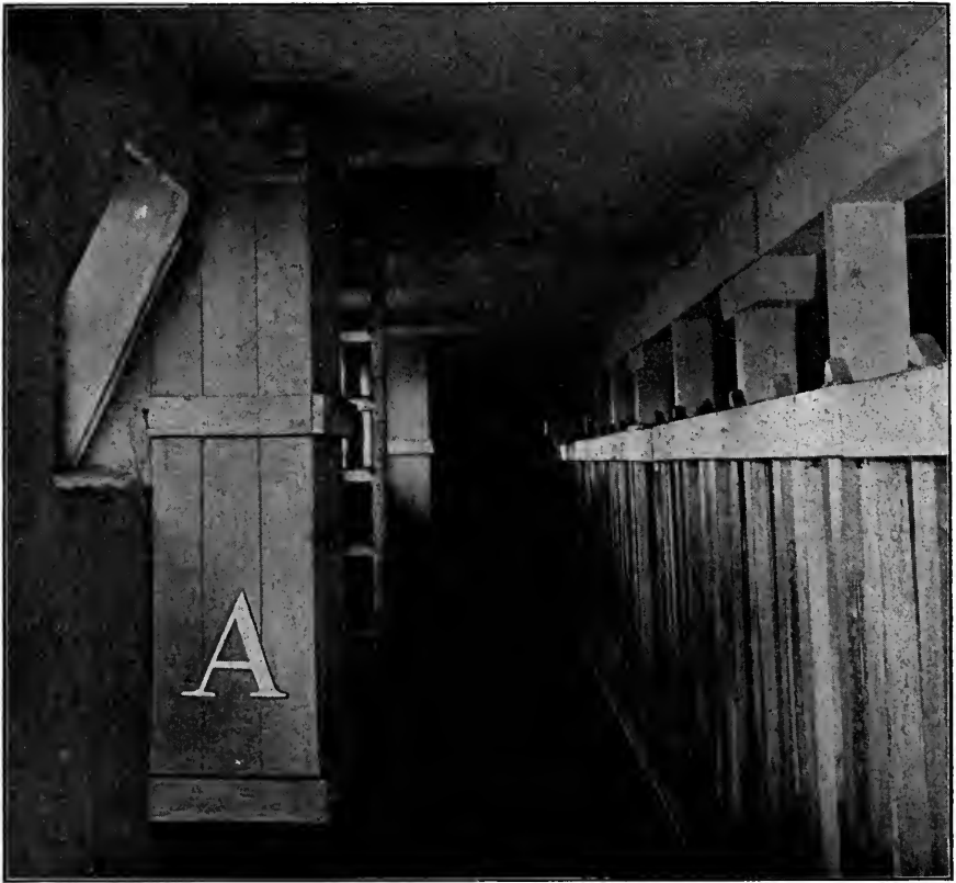
CUT 21. THE KING SYSTEM OF VENTILATION IN DAIRY BARN, SHOWN IN CUT 20. FRESH AIR IS CARRIED BETWEEN JOISTS OVERHEAD TO CENTER OF BARN; FOUL AIR DRAWN OUT FROM NEAR FLOOR BY FOUR LARGE VENTILATORS CARRIED ABOVE ROOF, CAUSING A CONTINUOUS CHANGE OF AIR WITHOUT CREATING A DRAFT ON THE COWS. VENTILATOR SHOWN AT "A."
