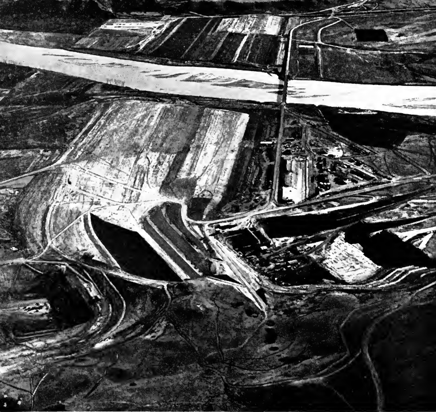
10. Garrison Dam on the Missouri River, North Dakota. Outlet works will go under the curving portion of the dam in the foreground.
